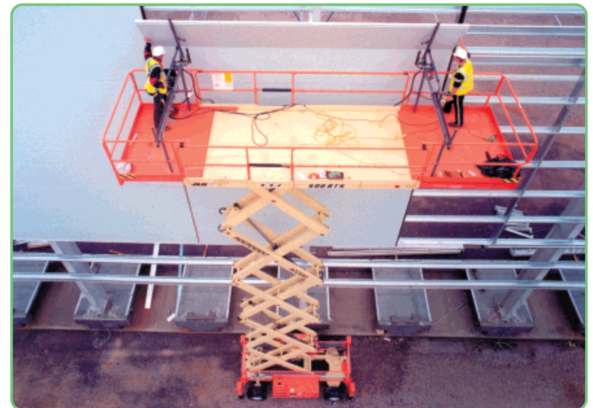
Figure 9. Insulated panels installed on a large coldstore
