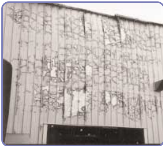
Figure 16. The fire rated (PIR) insulated panel wall cladding remained intact in this major fire although the internal roof structure behind had totally collapsed
